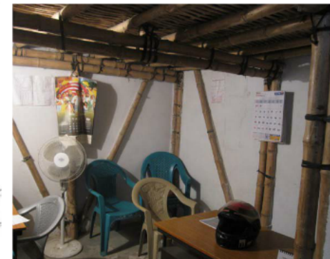
Figure 13: Diagonal braces for earthquake safety
